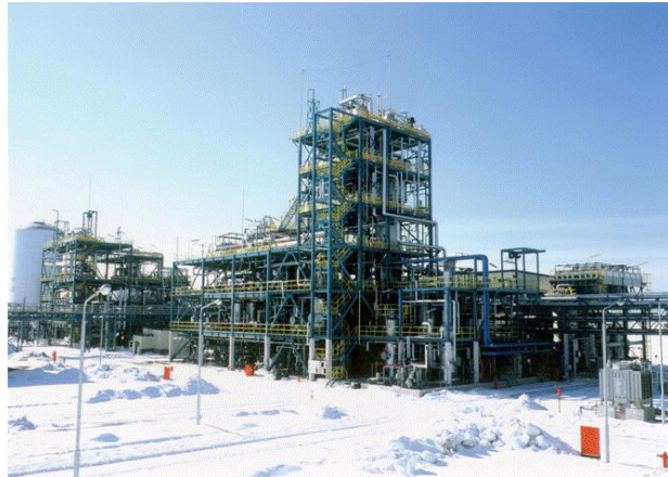
Figure 5. DME 100 tons/day Demonstration Plant
