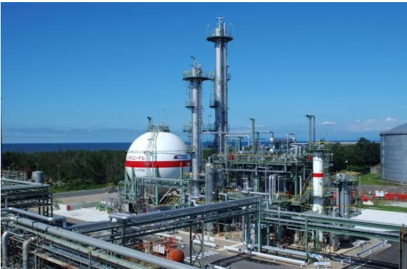
DME plant in Niigata
