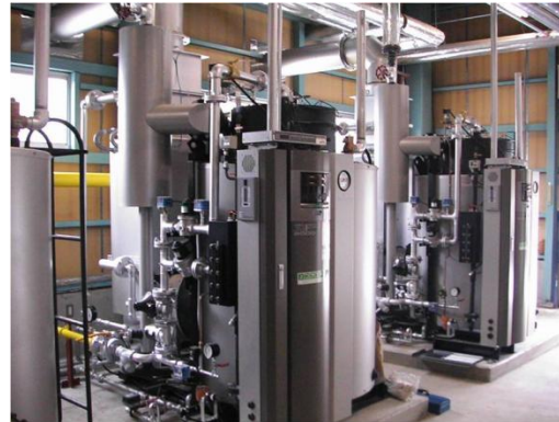
Boiler in Ichimasa
